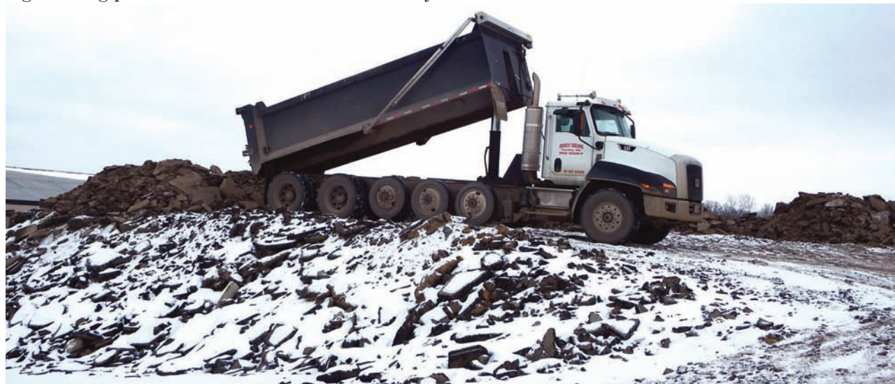
One of the 100 plus loads of asphalt tear out that was expected to be brought in on the day of our visit, arrives at the top of this stockpile of material and is dumped in a safe location.
